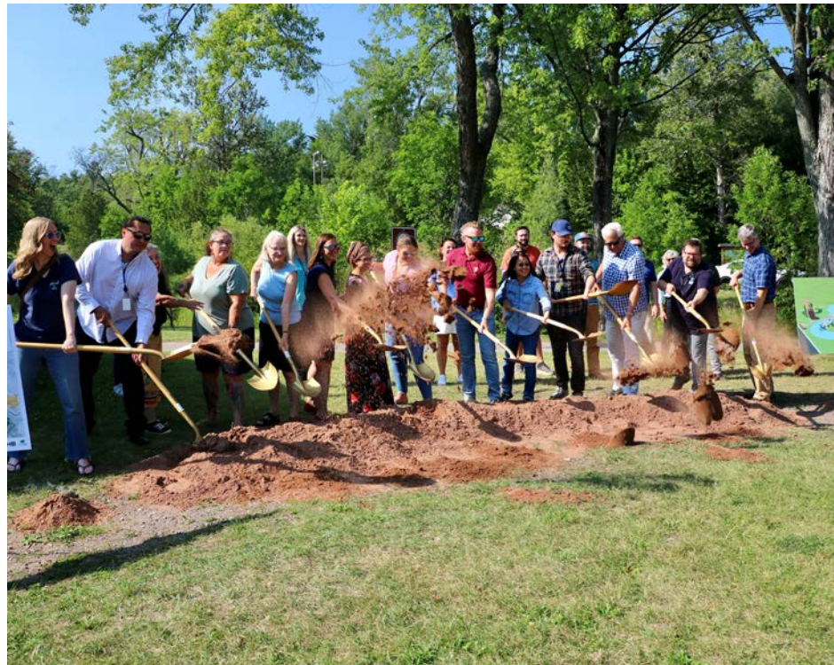
The Lincoln Park Ground Breaking event demonstrates the community collaboration and support involved in planning the improvement project.
