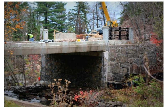
Improvements seen in the interactive map tool include on-gong improvements to the Chester Creek Bridge
