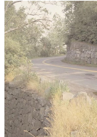
These stone walls at Chester Bowl are in need of repair.
