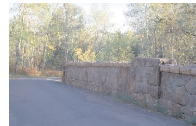
Native stone is used along the entire parkway in bridge and wall construction.
