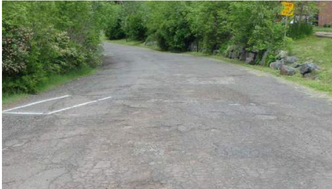
Roadway paving and shoulders in poor condition throughout park
