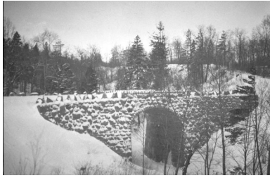
Stewart Creek Bridge in snow, date unknown. Source of photos this page: Northeast Minnesota History Center, UMD.
