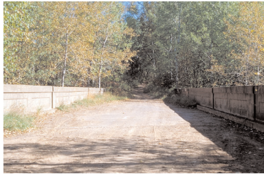
The railroad bridge carries the Mission Creek segment over the Munger Trail.
