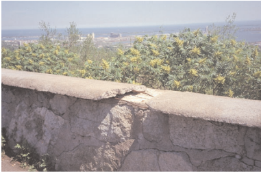
This rock wall at an overlook near 28th Ave. W. is deteriorating.
