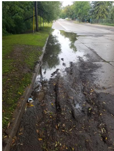
Clogged inlet at MS-2
