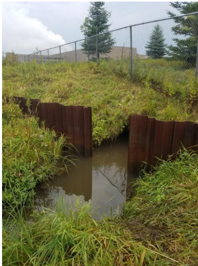
Inlet from paper plant at MS-1
