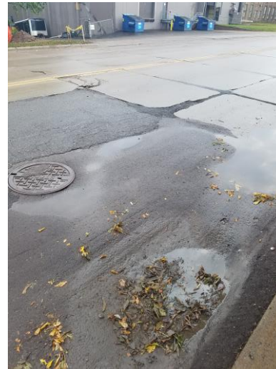
Clogged catch basin at MS-1
