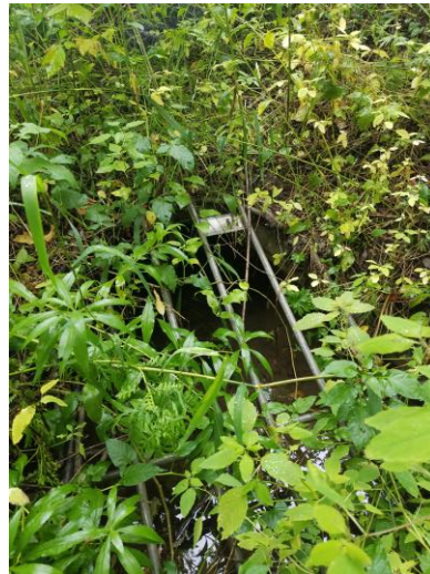
Inlet from wetland at MS-1
