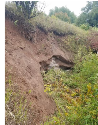
Bank erosion at top of MS-2
