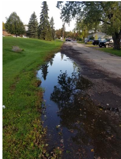
Ponded water that drains to T-2
