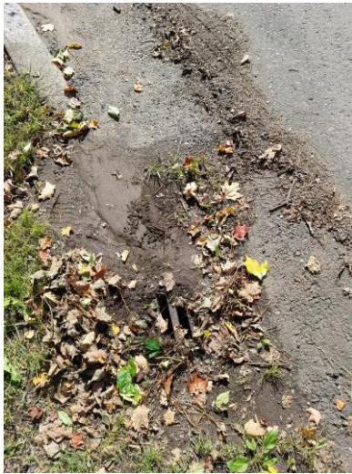
Clogged catch basin at MS-5
