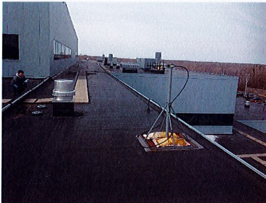
Observation #1 Most of the field seams have been overlaid. There are still quite a few curbs and edge flashing to address
