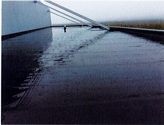
Observation #1 All the field seams have been stripped in on this section
