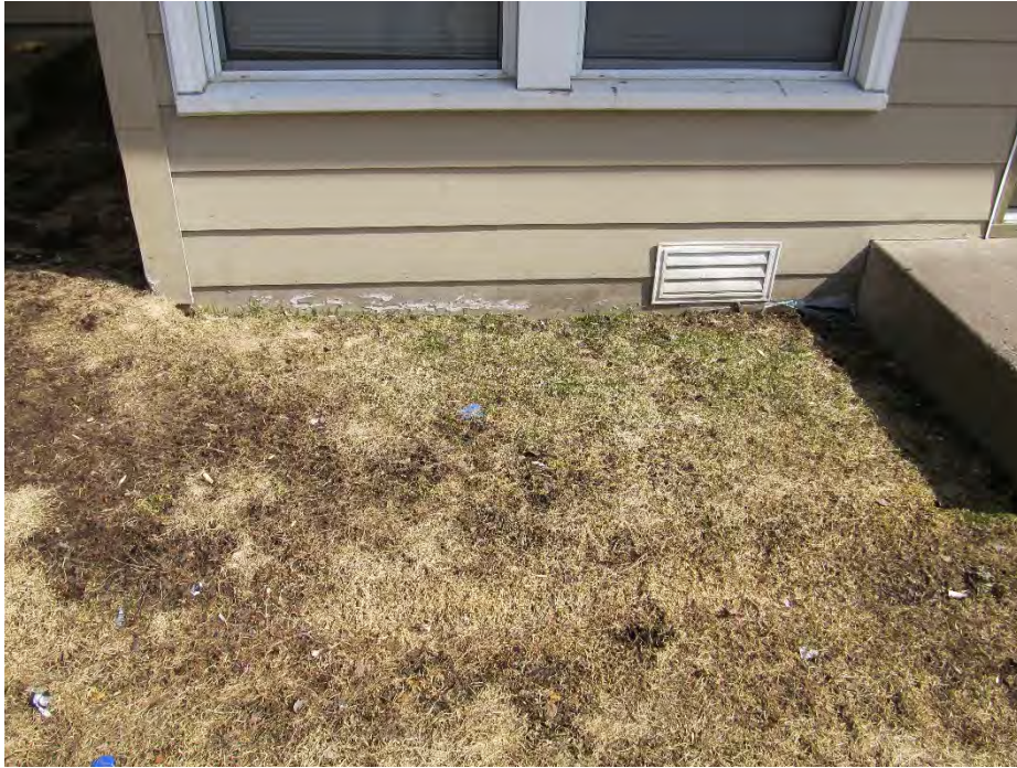
Figure 5 Fiber cement into the soil and at uphill location. Note typical deterioration of siding at this location
