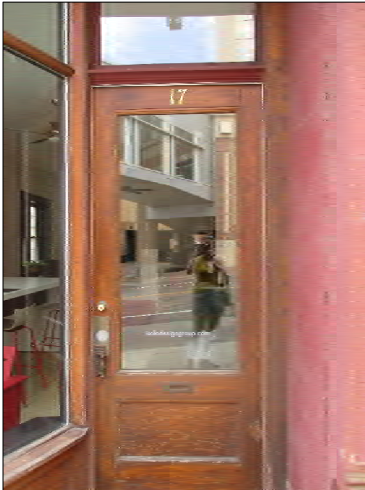
Photograph 16: View of a typical historic wood panel door in a commercial storefront with some of its original hardware.
