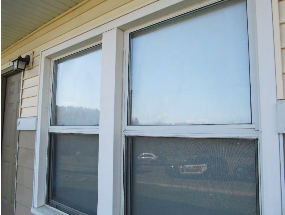
Figure 7 Fogged thermopanes in newer window series
