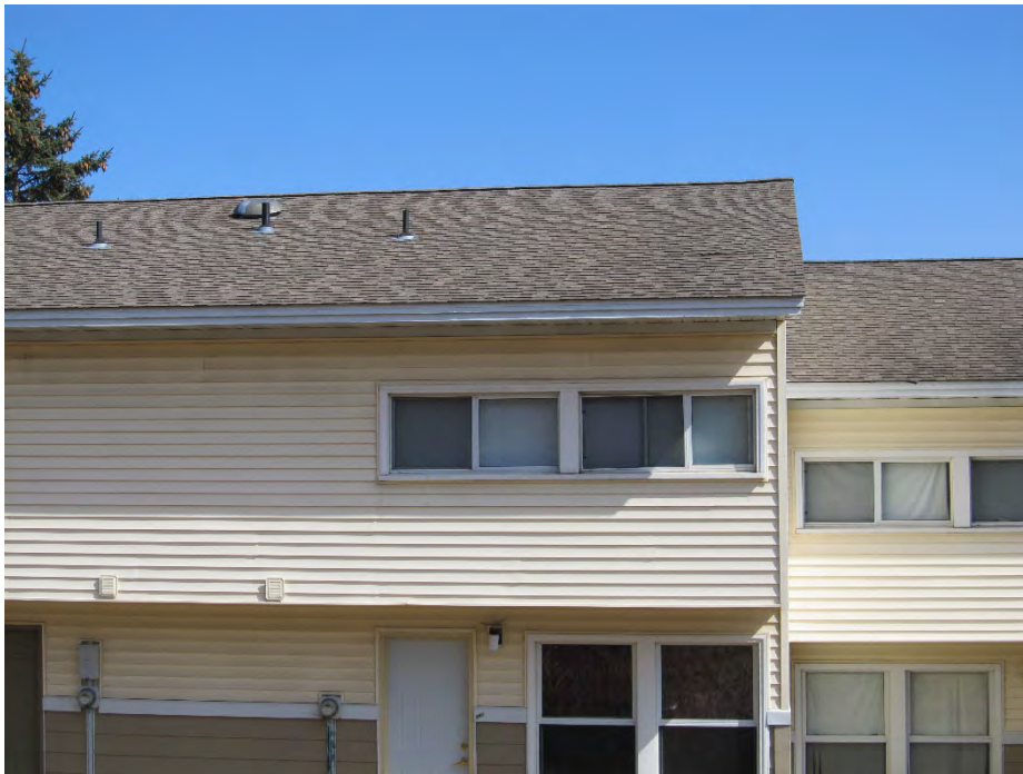
Figure 2 Typical roof picture. Note shingle damage, otherwise good conditions
