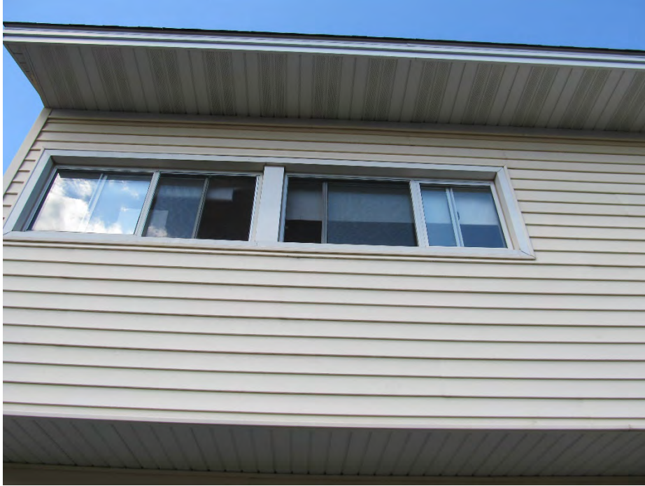
Figure 3 Soffit and trim in good condition as us upper siding of vinyl.
