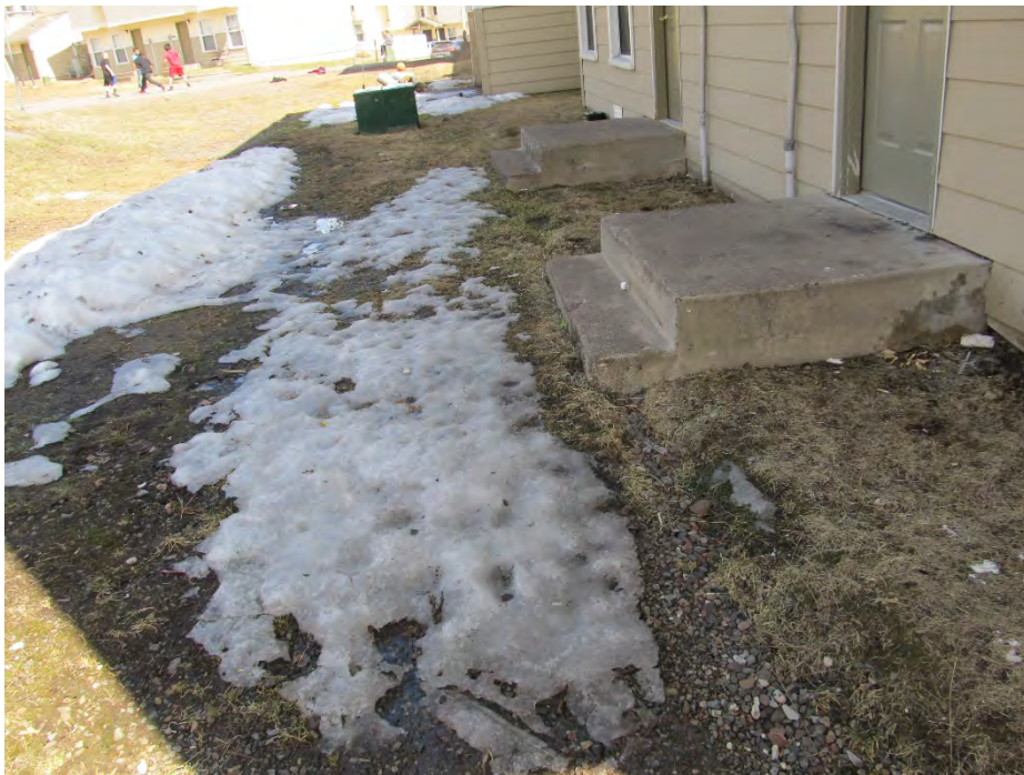
Figure 10 Stoop condition, solid but some grease stains
