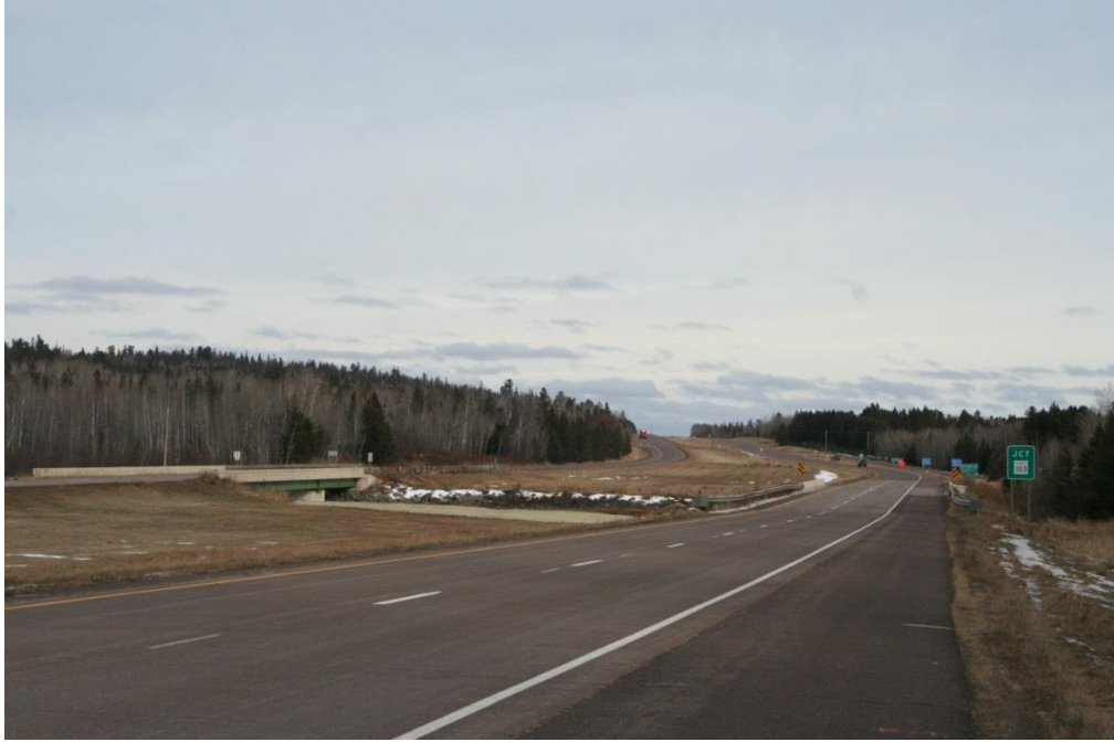
Figure 4. Knife River Bridges (Br. No. 9341, ST-DUL-009, and 9339, ST-DUL-008), view facing east. The bridges were widened in 1998 to allow for a continuous 8-foot shoulder on TH 61.
