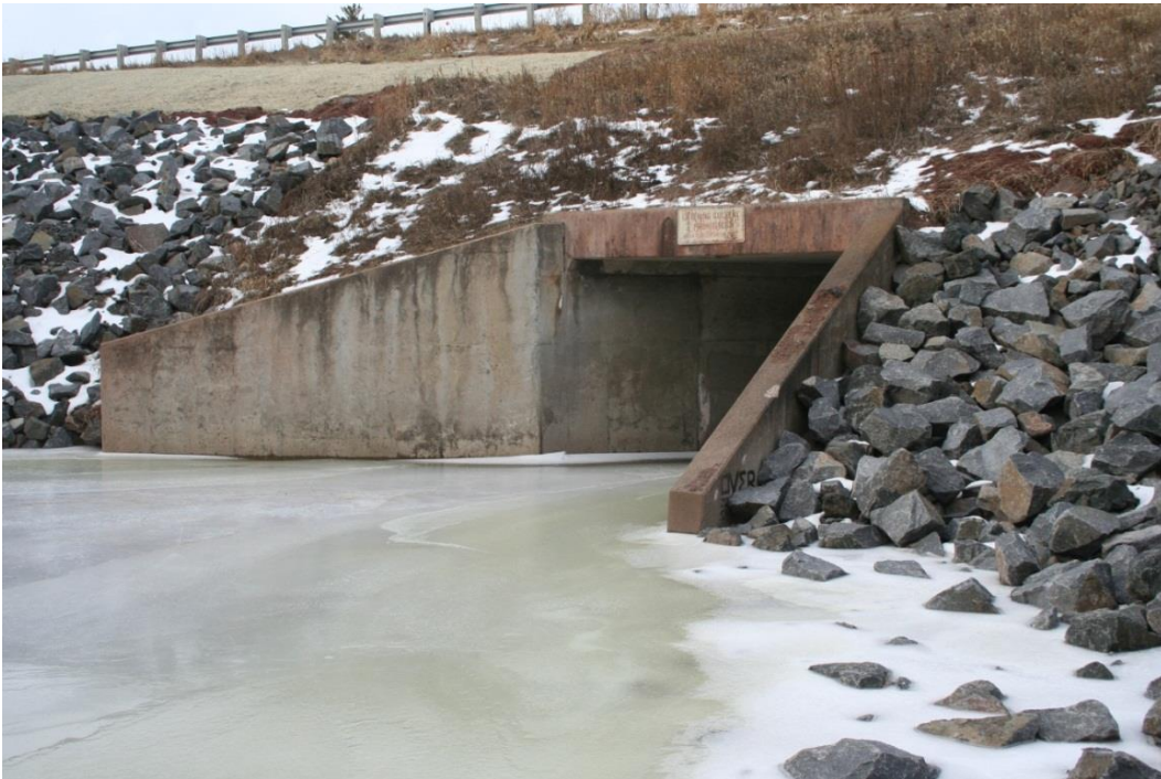
Figure 19. Typical concrete box culvert and guardrail (background) along TH 61, view facing northwest. This box culvert is located at the Sucker River. Rip-rap replaced after regional flooding in 2012.
