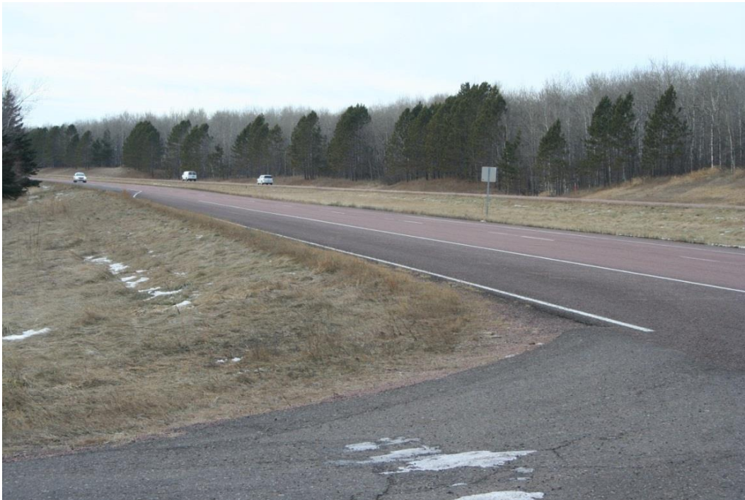
Figure 15. Typical turn lane along TH 61, view facing west. Turn lane located at North 78 th Avenue.
