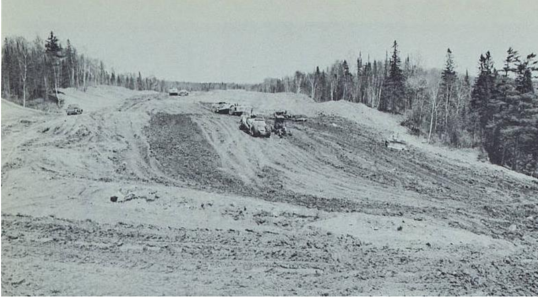
Figure 10. "Four-lane grading near the French River on the new North Shore right of way between Duluth and Knife River." Minnesota Highway Department, Minnesota Highways , June 1960, available at http://reflections.mndigital.org/cdm/compoundobject/collection/mdt/id/2324 (accessed 24 January 2013).
