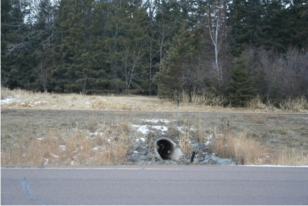
Figure 18. Typical concrete pipe culvert in the center TH 61 median, view facing north.
