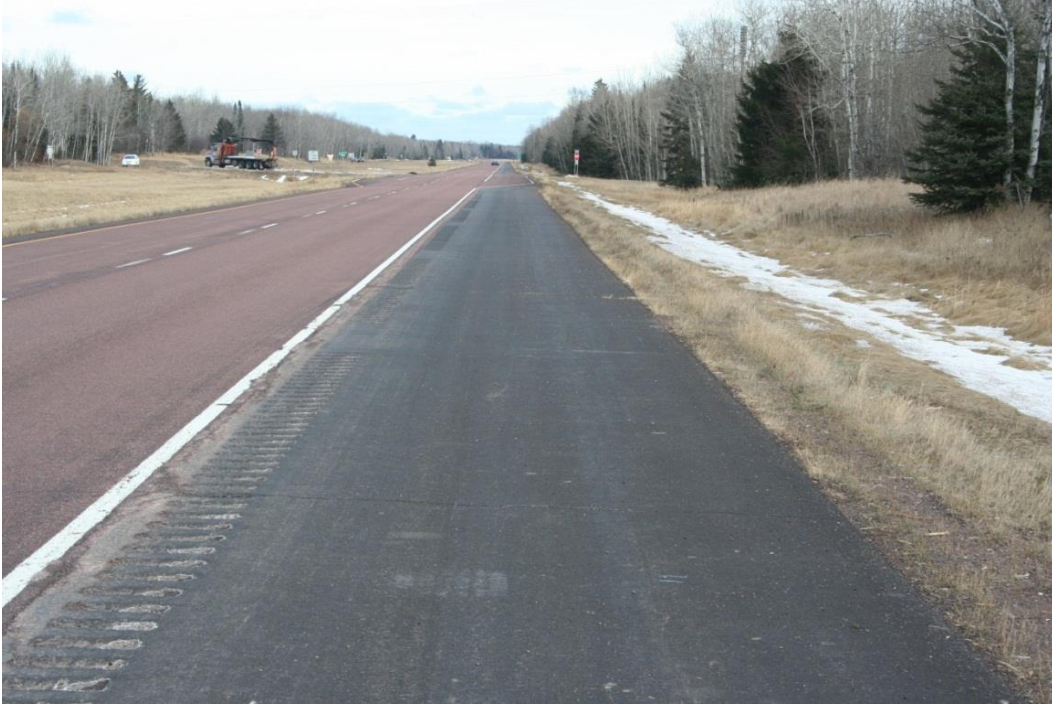
Figure 16. Detail of the outside 8 foot bituminous shoulder along TH 61, view facing east. Note how turn lanes utilize the shoulder, as seen in the background.
