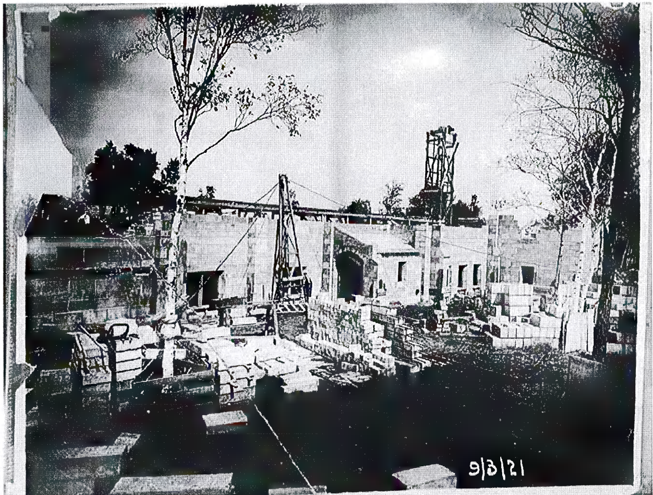
Figure 4. United Protestant Church construction progress in September 1921. Photograph courtesy of United Protestant Church.
